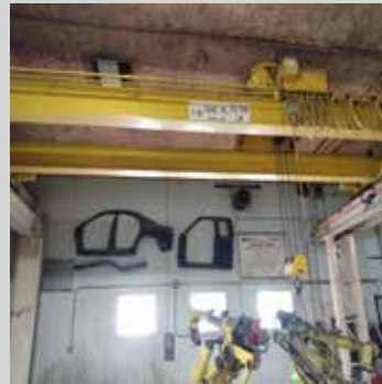
15 Ton R-M Overhead Crane 30' Width
