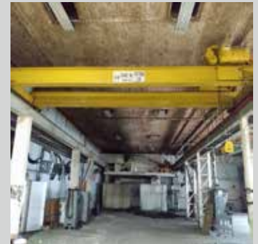
15 Ton R-M Overhead Crane 30' Width
