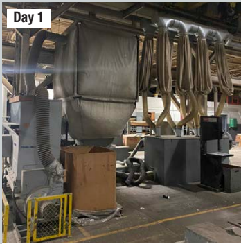
Foam Reclamation Unit
